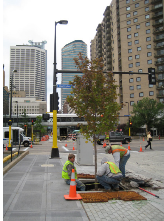
Pervious pavers route stormwater into the Silva Cell system.
