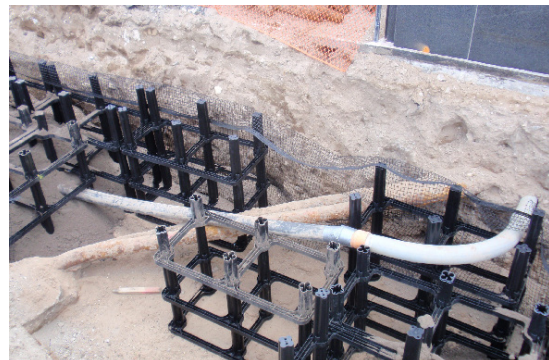
Silva Cells accommodate new and existing utilities.
